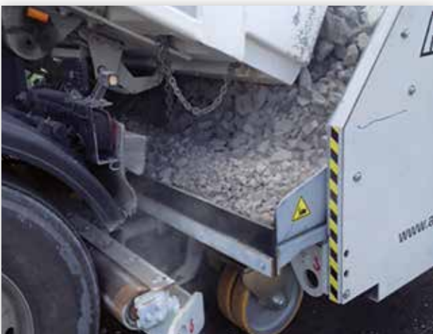
Loading process with hydraulic lift adjustment of the bunker flap
